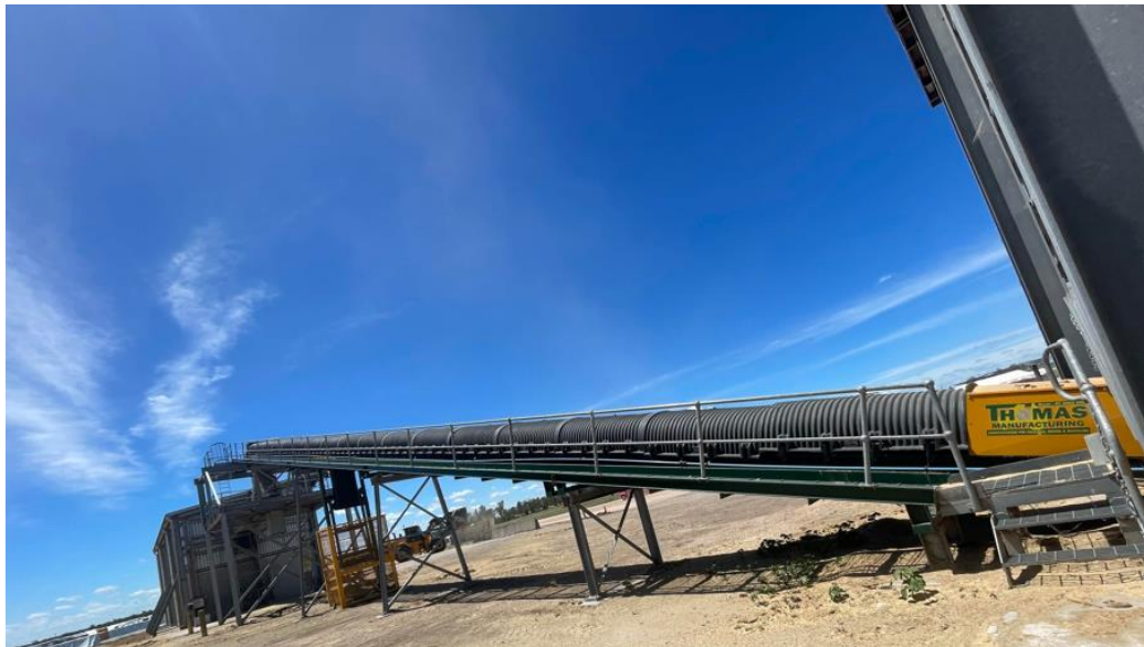
Figure 2: Conveyor System Replacement of Chain with Belt
