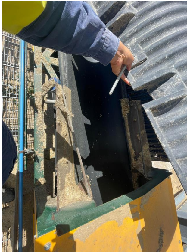
Figure 3: Inside the Conveyor Belt System
