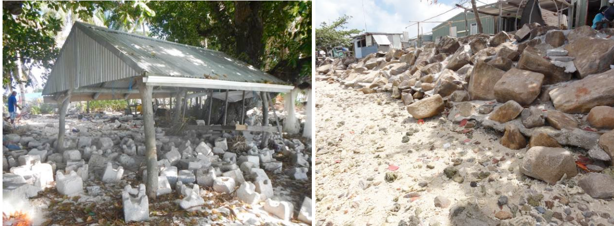
Figure 5 Sand and modified cube armour blocks deposited through community of Nukulaelae after TC Pam, Tuvalu (Source PWD GoT); failed seawall on a sand starved beach on Iama, Torres Strait.
